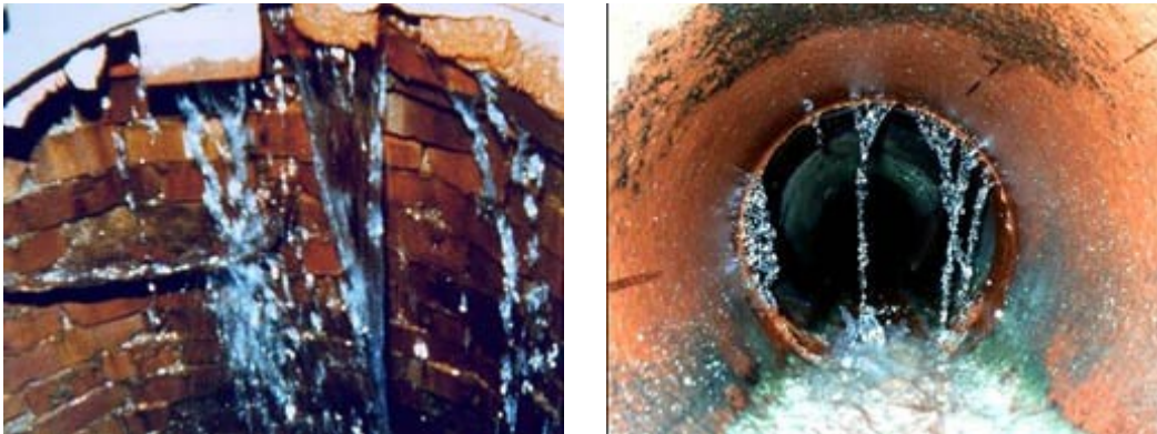
Figure 1. Stormwater entering into the sewer system from a manhole, at left, and from a defect inside a pipe, at right.
