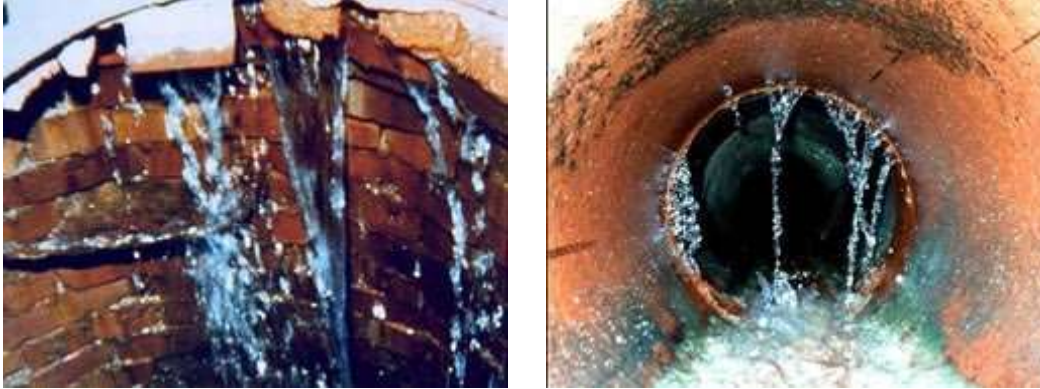
Figure 1. Storm water entering into the sewer system from a manhole, at left, and from a defect inside a pipe, at right.
