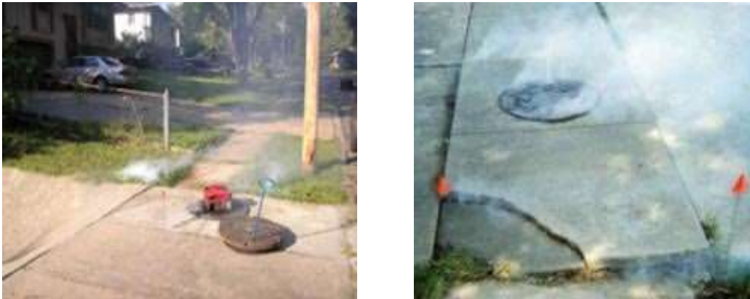
Figure 2. capacity blowers are used to pump non-toxic smoke into a manhole (left photo). In the right photo, smoke is pushed into the system and emerges from cracks in the sidewalk and at a downstream manhole.
